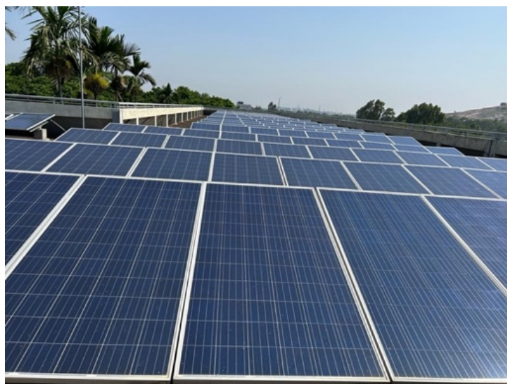
Fig 3.1. Actual Field Image of the PV facility of 125kWp at Bengaluru, Karnataka
