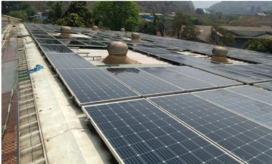
Fig 3.5. Actual field Image of 191.9 kWp at Khopoli, Maharashtra
