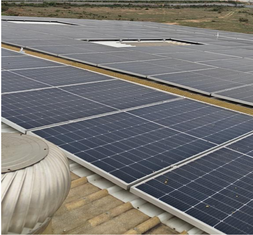
Fig.3.9. Actual field Image of 235 kWp at Maheshwaram, Telangana
